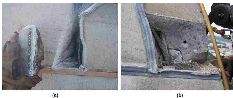
Figure 5.4. Spalling of pyramidion panels of the Washington Monument: (a) North face, (b) Northeast corner (Wiss, Janney, Elstner Associates, Inc., 2011)
